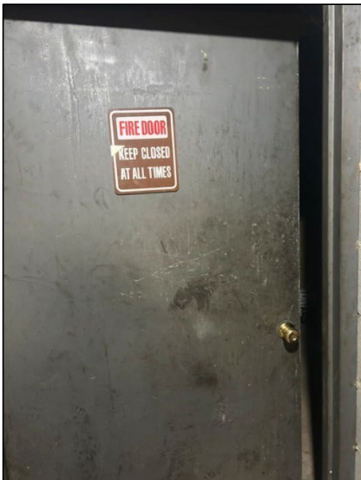
Damaged Fire Door in Basement Space
