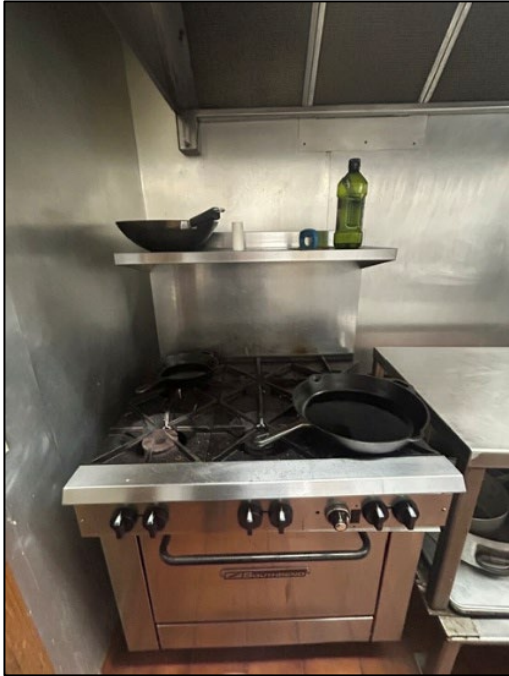
Commercial Range Under the Hood in Kitchen
