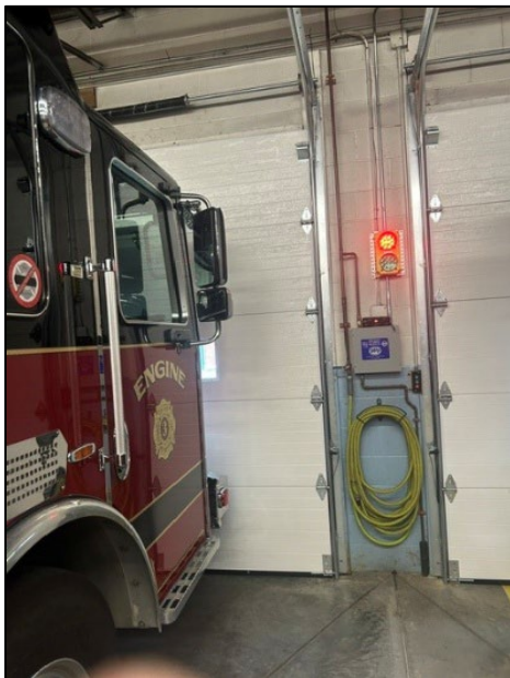
Traffic Style Signal System Controlling Safe Exits from the Apparatus Bays
