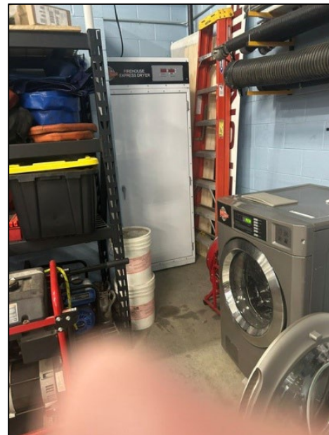
Gear Extractor and Gear Dryer in Apparatus Bay
