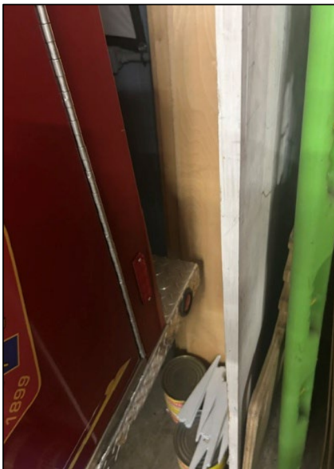
Very Limited Clearance of Apparatus Tailboard to Cabinets in Bay
